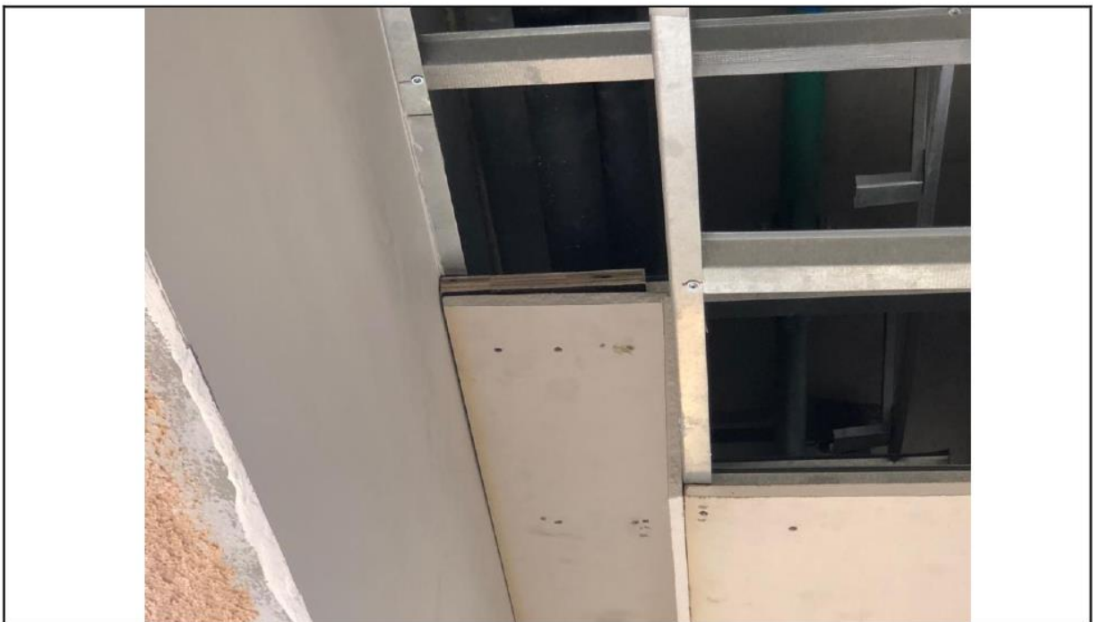
Ply wood to be fixed properly
